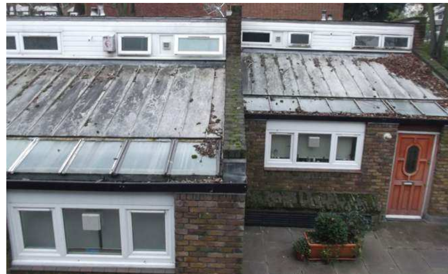
Some are in the better conditions than others are due to be replaced in 2015 by the Lambeth Council.
