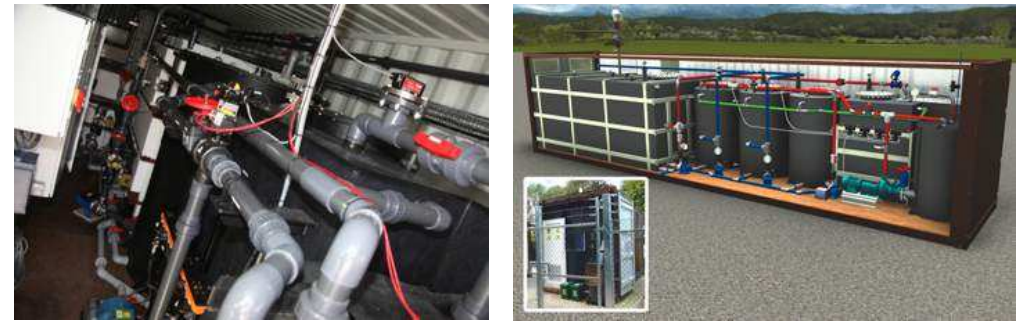
Anaerobic digester plant – compact installation
